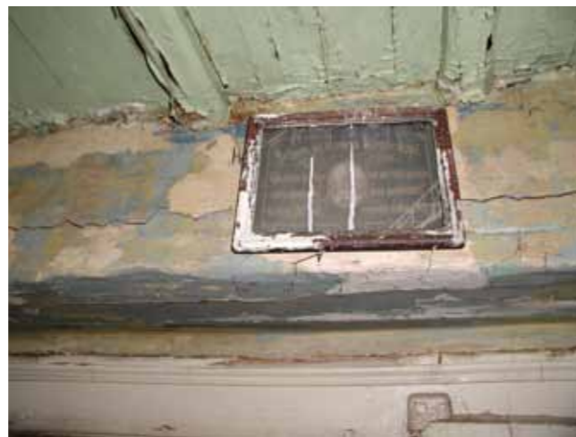
Figure 4.1.1.6: Timber joist ceiling with apparent deformation of its elements. Sources: M. Drdäcký.
