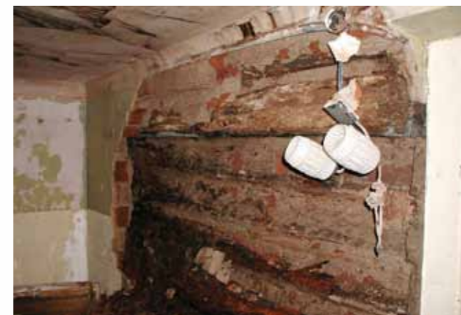
Figure 4.1.1.1 Log wall discovered after destruction of a brick veneer. Source: M. Drdäcký.
