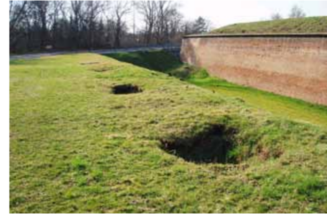
Figure 4.7.1.4: Sunken soil over a failed vault. Source: Roman Gazsi.
