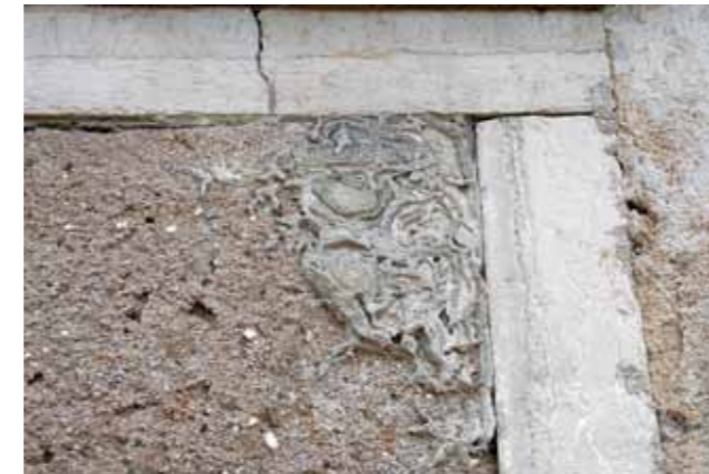
Figure 4.7.2.7: Sulphate corrosion of the façade plaster. Source: ZAG.
