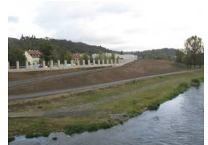
Figure 4.2.3.10: Originally designed as a solid wall - modified after pressure from LA, Source: T. Drdäcký.
