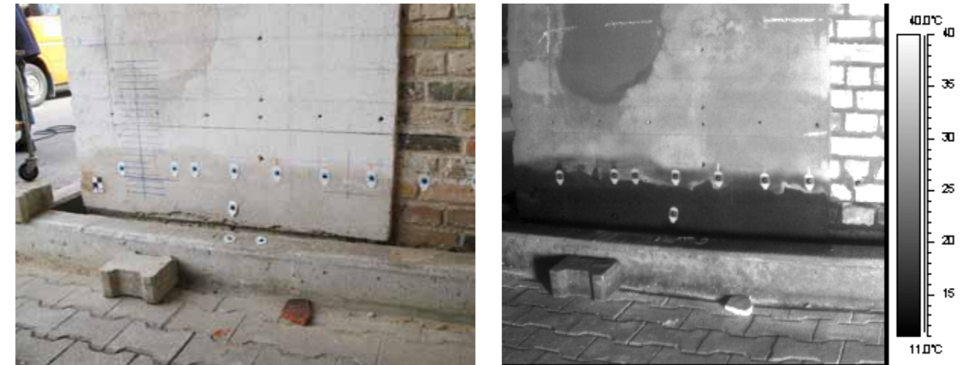
Figure 7.4.3.1: Photograph of a brick masonry specimen section partly covered with plaster (left). The specimen is contained in a concrete basin and was flooded with tap water. In the reflection thermogram recorded after 5 min. of heating, two moisture horizons can be clearly differentiated (right). Source: BAM.
