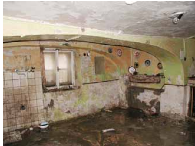
Figure 4.1.1.5: Deflected flat arch with an open crack decreasing the safety of the ceiling and requiring strengthening repairs. M. Drdäcký
