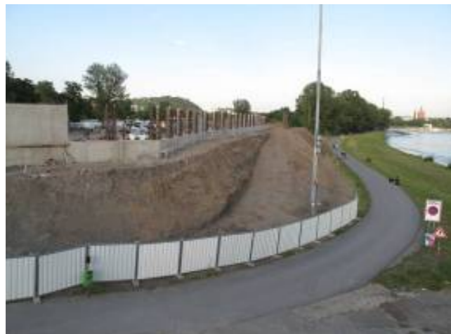
Figure 4.2.3.15: New mound and wall, compared to the human scale. Source: T. Drdäcký.
