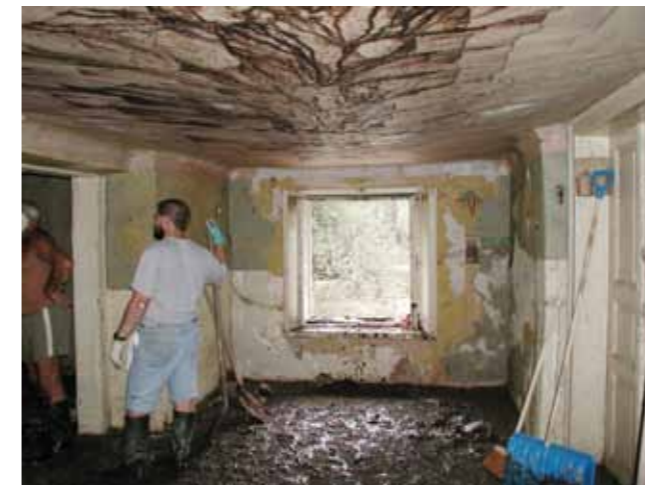
Figure 4.1.1.8: The exceeded deflection of the timber ceiling is well visible, as is the soiling of the building with mud. Sources: M. Drdäcký.
