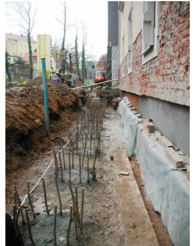
Figure 3.1.4.2 (above): Gabion walls in Romania to prevent damage from the annual spring flood. Source: BAM.
