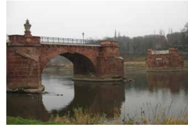
Figure 4.2.4.6: The famous Pöppelmann Bridge in Grimma: destroyed during the Mulde flood, 2002. Source: BAM.
