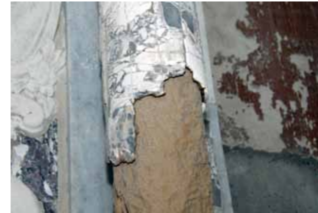
Figure 4.7.2.5: The elaborate work of Venetian stonemasons has deteriorated into fragments. Source: ZAG.
