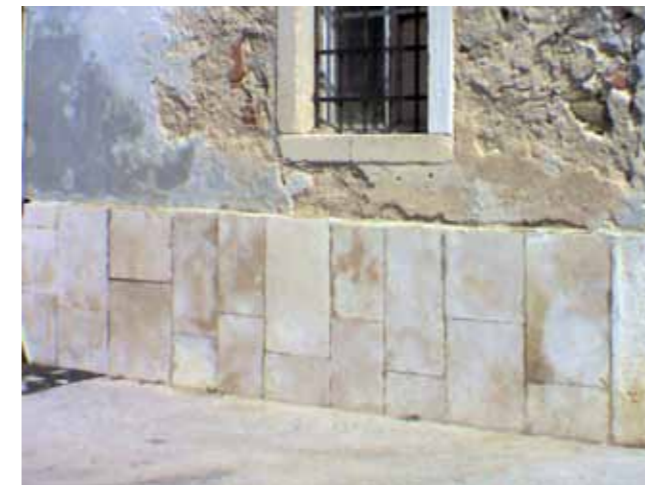
Figure 4.7.2.9: Degradation of the façade plaster on the west façade, caused by the capillary rise of groundwater. Source: ZAG
